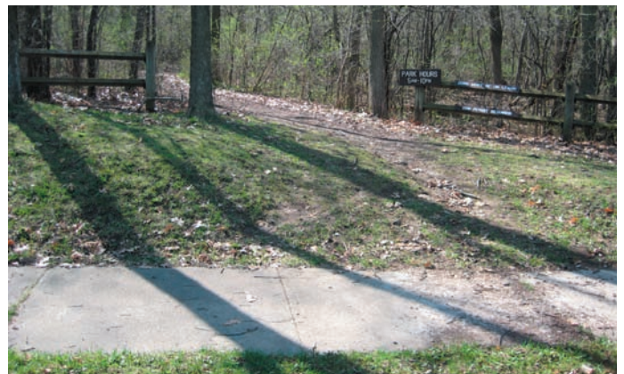
Erosion from Stormwater Runoff is an Issue
