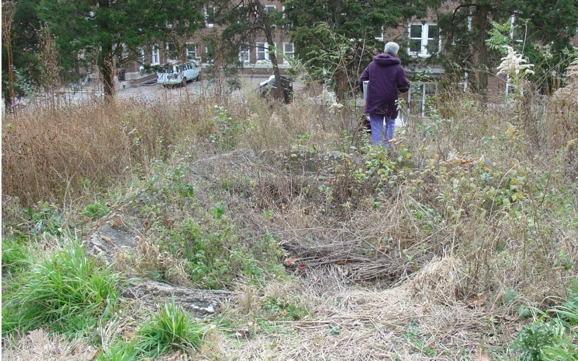
Figure 3- 52: Remnant of cement retaining pond on hill north of main Sanatorium building, 2010. (source: QEA 7589)
