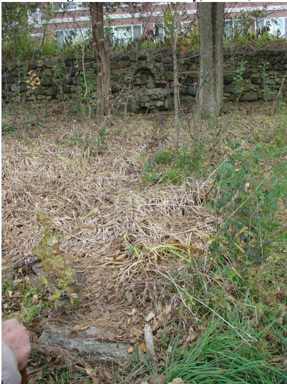
Figure 3- 25: Grotto in retaining wall south of Dormitory and remnants of cement drainage channel, 2010 (source: QEA 7595)
