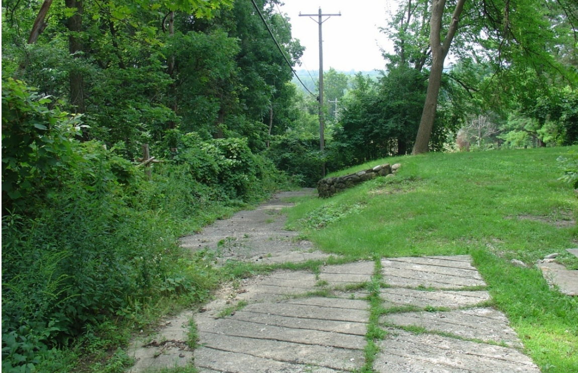
Figure 3- 34: Remnants of service drive and stone retaining wall on east side of Dormitory (source: QEA 6222)
