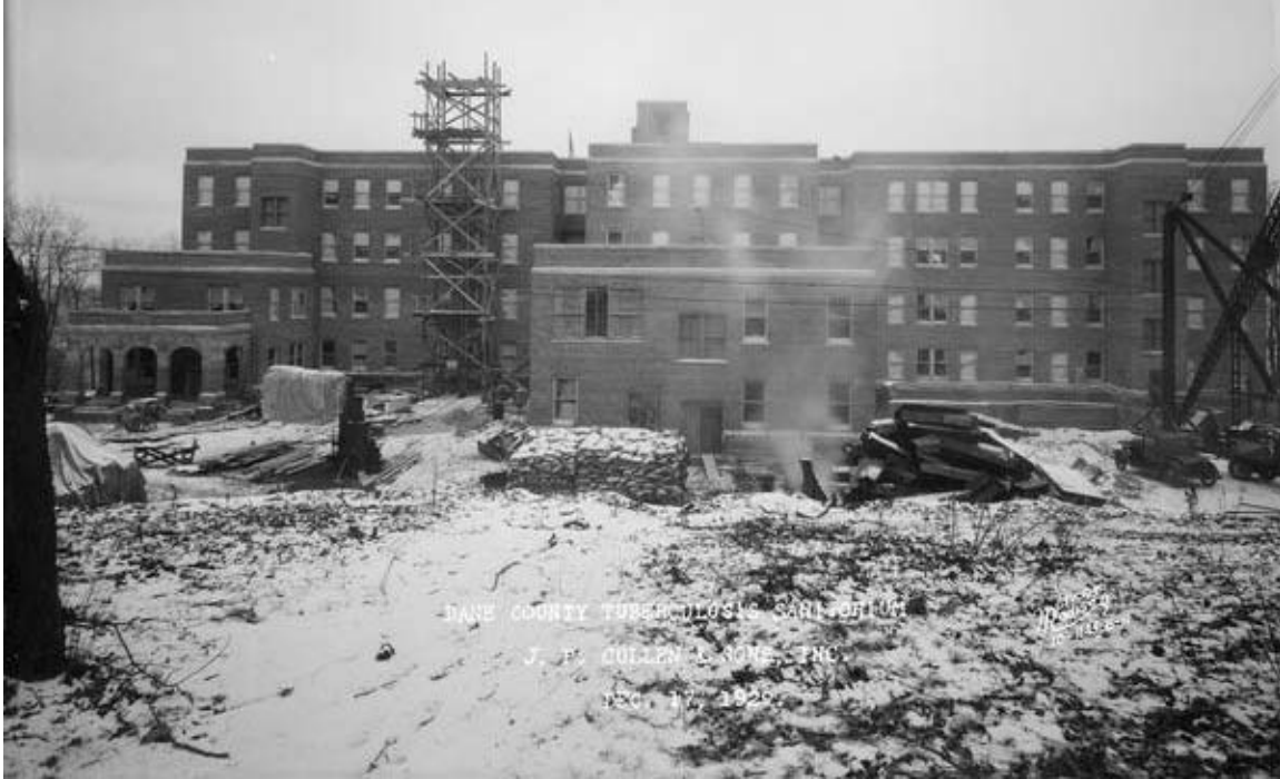
Figure 2- 5: North side of Lake View Sanatorium under construction, 17 December 1929. (source: Wisconsin State Historical Society Archives, 21161, by Angus B. McVicar).
