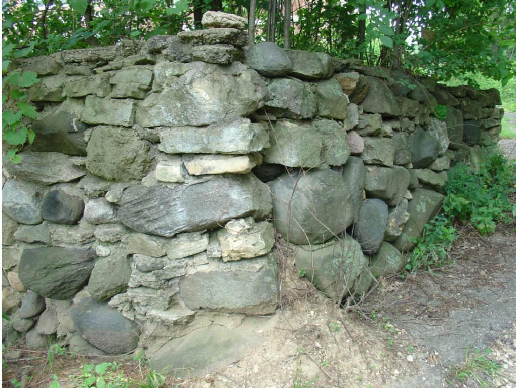
Figure 3- 24: Material is washing out from behind the southeast corner of the retaining wall and undermining its structural stability, 2010. (source: QEA 6263)
