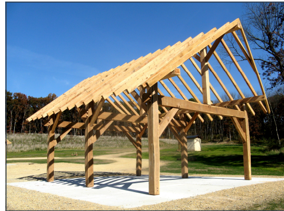
Frame of new shelter at Scheidegger Forest. Wood used for construction of the shelter was harvested from Scheidegger Forest
