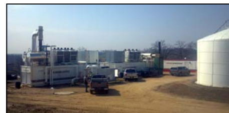
Two generators provide enough electricity for 2,500 homes. A liquid storage unit is on the right.
