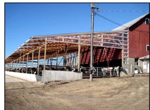
In compliance with Chapter 14, a roof installation covers the feedlot and prevents manure runoff into local surface waters
